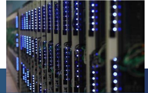
Data Center & Storage
